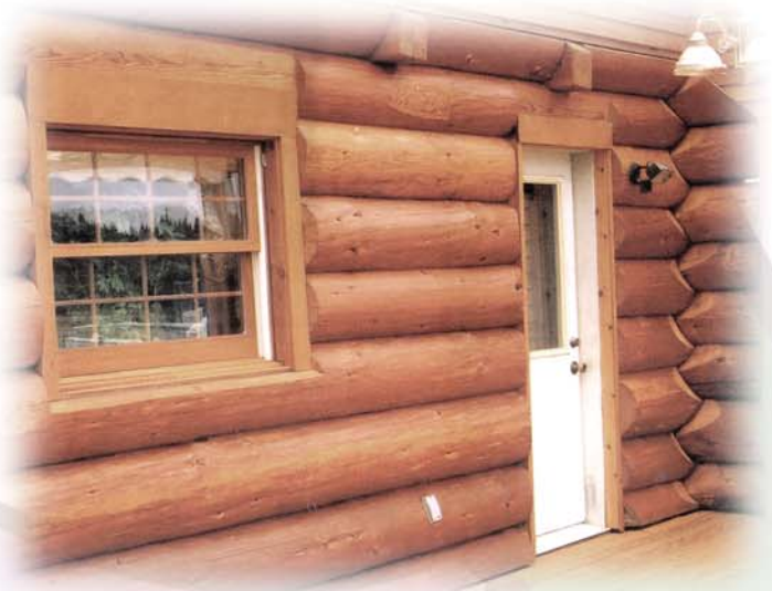
Above: Before and after Strip & Brite applied on the weathered wood of this log home
